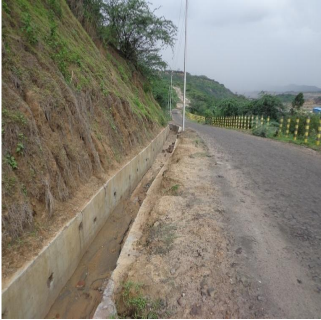
Plate -5: Catch drain all along the approach road
